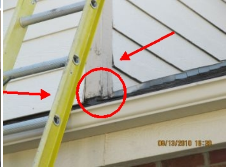
Loose siding, trim weathering
