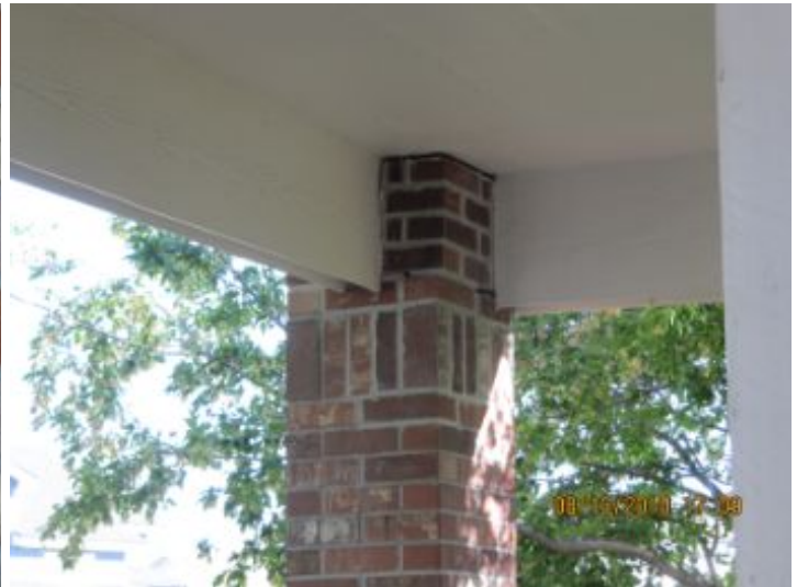
Column has settled, top portion of brick loose
