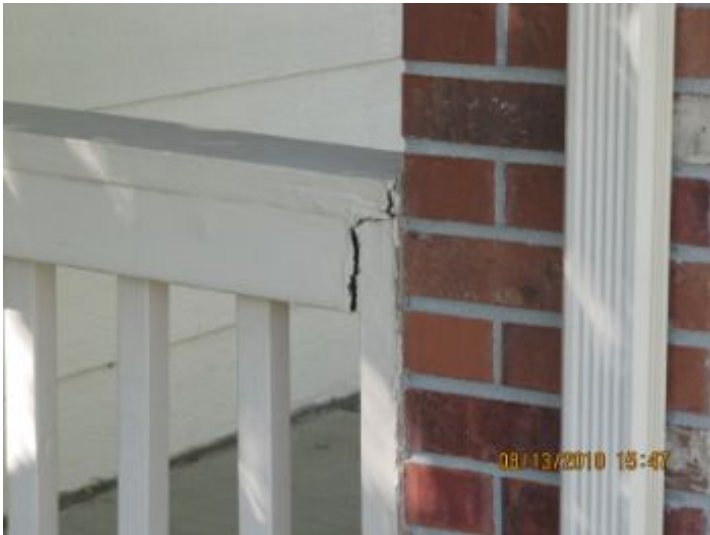
Railing pulled apart, needs caulking
