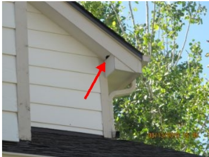
Hole where squirrels gained access to attic
