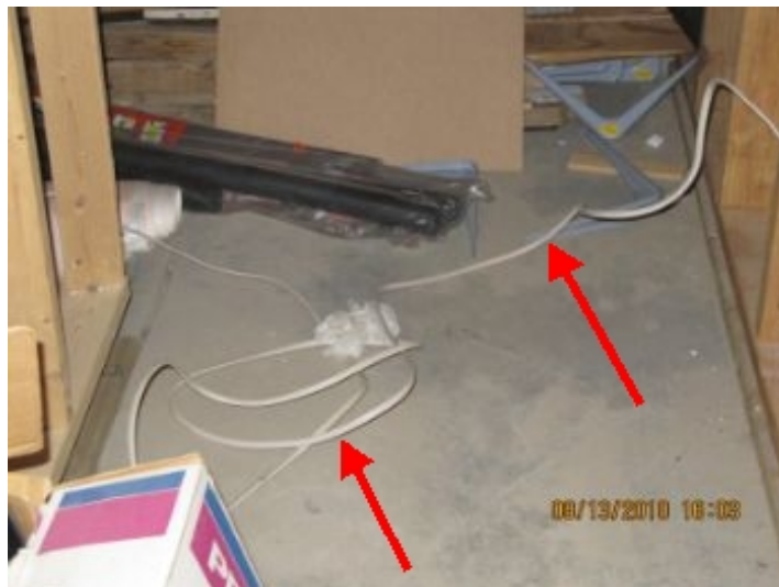
Wiring needs to be secured to framing and protected
